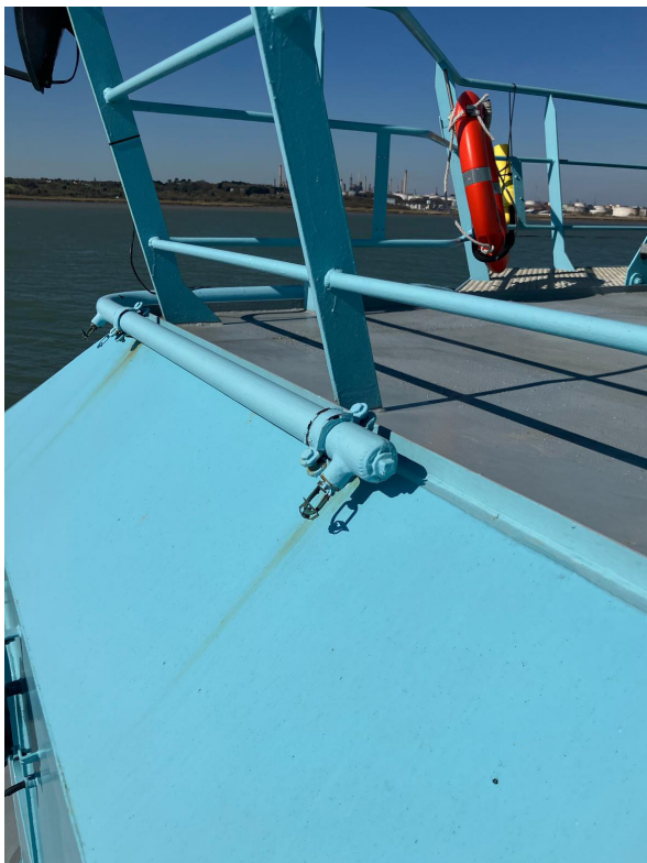
Accommodation drench system
